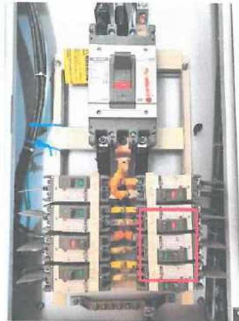
(The Main Distribution Panel Board)
