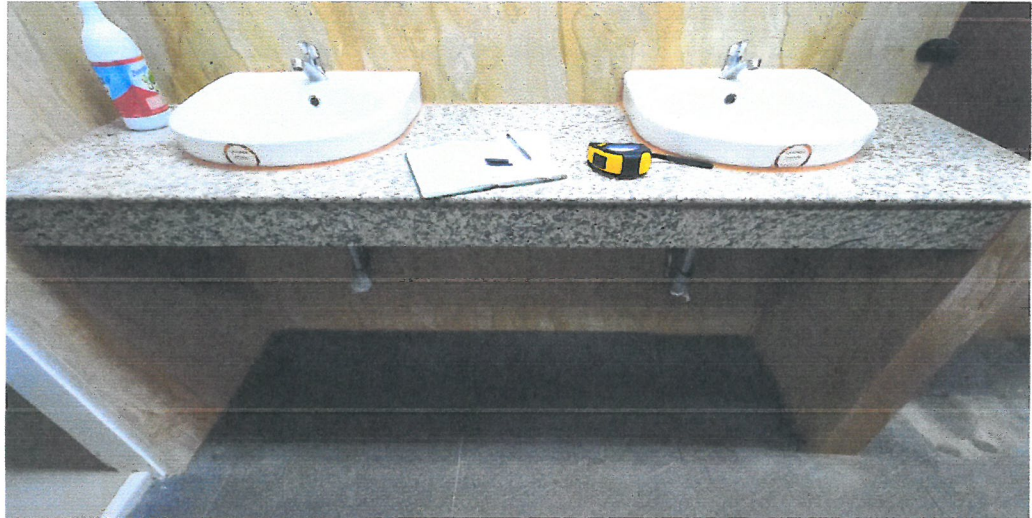
Two (2) sets of cabinetry with approximate dimensions: (Verify for Actual) Length = 1.70m, Height = 0.75m, Width = 0.50m
