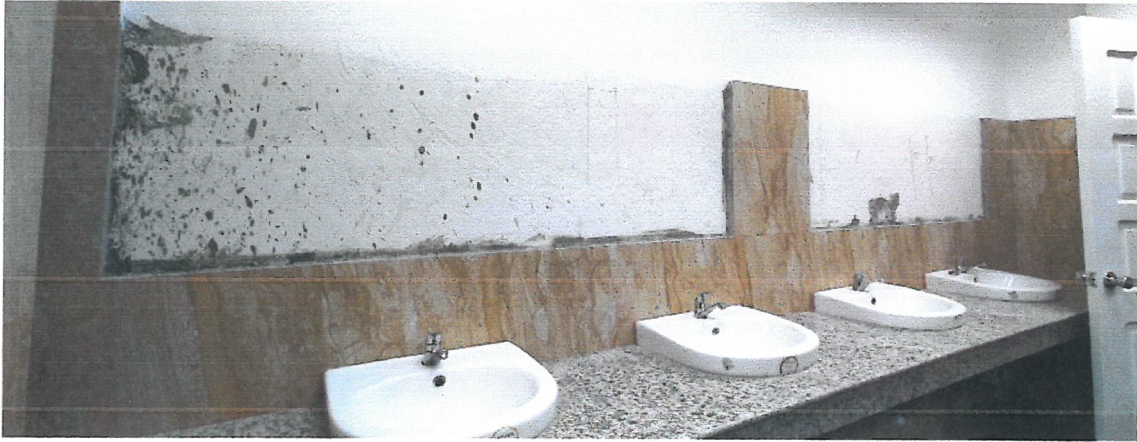
Two (2) sets of fixed mirror with approximate dimensions: (Verify for Actual at Women's Toilet) Length = 1.70m, Height = 0.60m (Left); Length = 1.50m, Height = 0.60m (Right)
