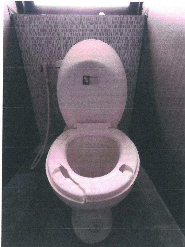
(a) Damaged Water Closet Cover
